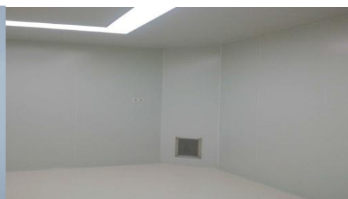
PROJECT CLEANROOM RSUD BOJONEGORO
