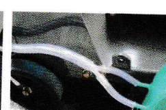
double water pipe for cooling both sides
